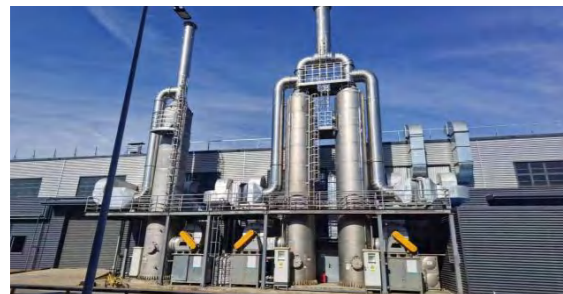
Exhaust gas treatment facility at the Yangzhou base
